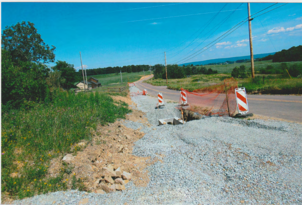
MUD PIKE CONSTRUCTION IN FRONT OF THE WEBSTER "BUDDY" AND ROBERT FOOR RESIDENCES
