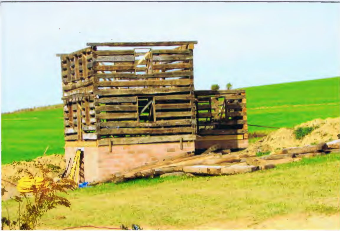
A SCENE IN OCTOBER 2023 OF ROGER AND SHERRY KALAHA'S LOG HOUSE BEING ERECTED AT THEIR STONYCREEK TOWNSHIP PROPERTY. THEIR LOG HOUSE ORIGINALLY WAS LOCATED IN THE BARD AREA OF BEDFORD COUNTY.
