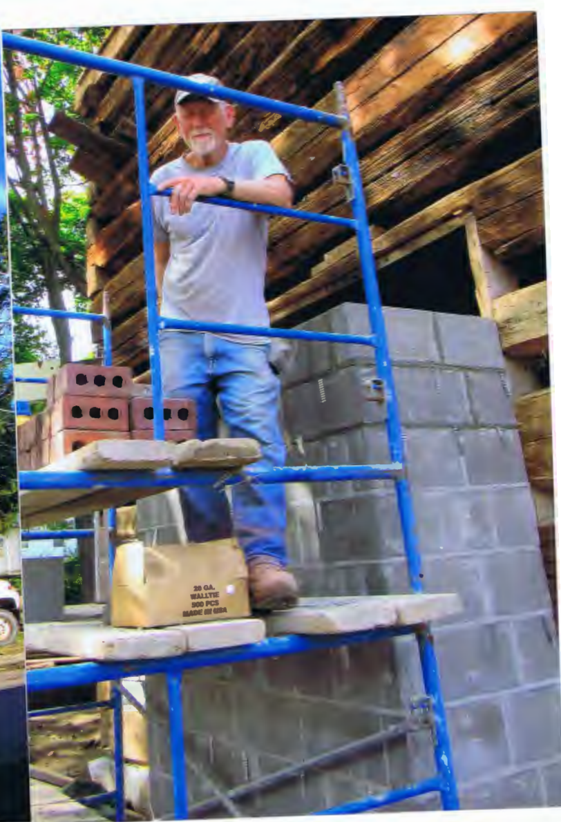
ALLEN LONG LAYING THE BLOCKS FOR THE CHIMNEY TO BE ADDED TO THE LOG HOUSE. OCTOBER 2, 2023
